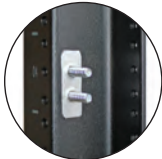
Ground Studs located directly on rack channel
