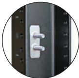
Ground Studs located directly on rack channel
